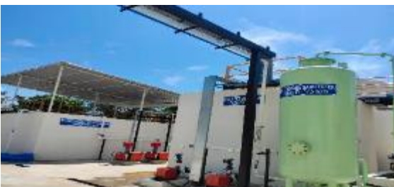
Multi grade sand filter
