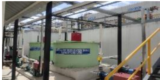
Lime slurry tanks-1&2
