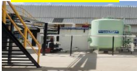
Multi Grade sand filter
