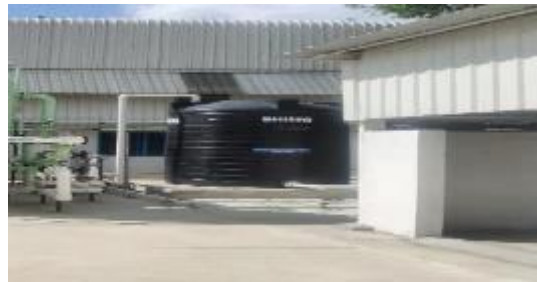
Treated water storage tank
